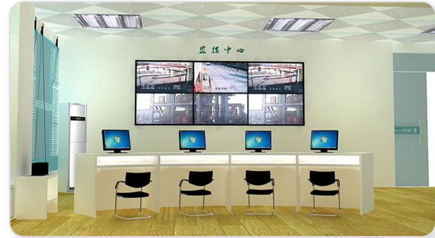
Smart Grid Monitoring Center
