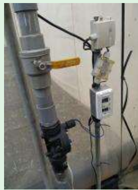
▲ The irrigation pipeline uses a controller and solenoid valve to automatically irrigate according to the light integral value
