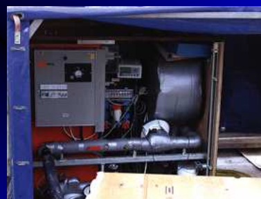
Thermal response test: measurement of effective heat conductivity of underground layers. Heated water will be pumped into u-tubes and inlet & outlet temperature will be measured.
