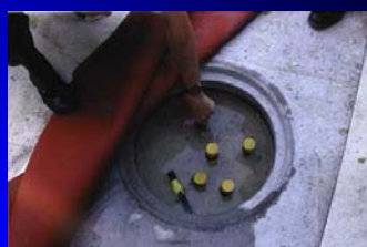
Surface top part of the borehole and double u-tubes. They will be connected to a heat-pump.
