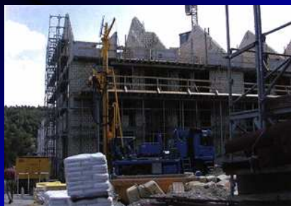
Construction of an apartment complex and a drilling machine for borehole heat exchanger
