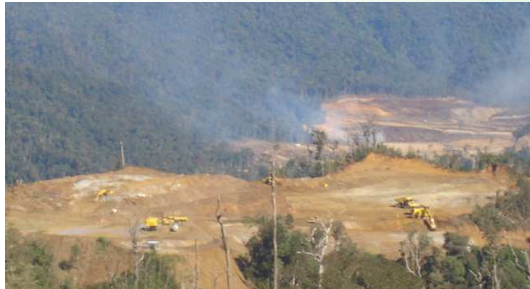
Increased construction related mine waste
