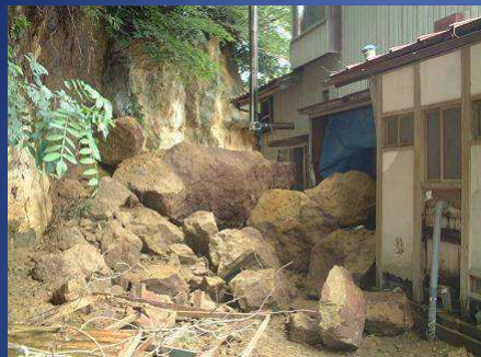
Slope failure caused by earthquake.
