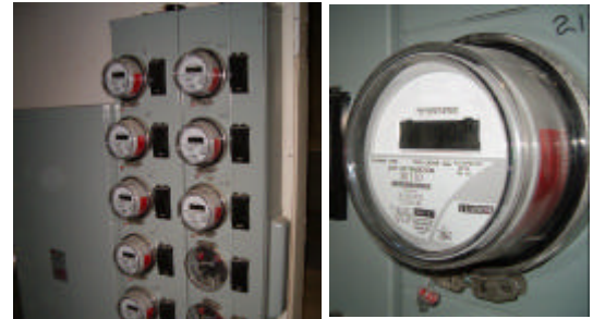
120/208v Network meters in an apartment complex
