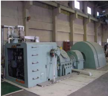
No.1 Steam Turbine (8,700kW)
