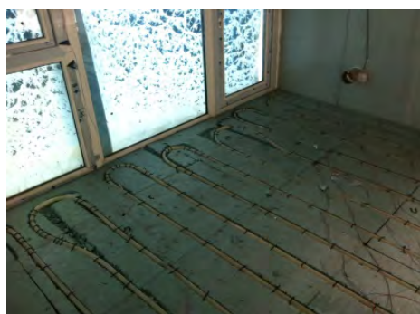
Figure 2 Hot water heating system
