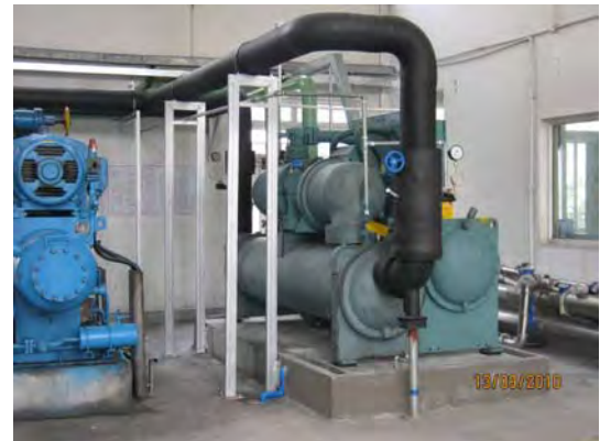
(a)170RT duplex conditions refrigerator
