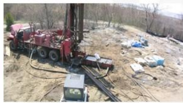
Ground Source Heat Pump
