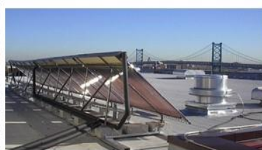
Solar Water Heating
