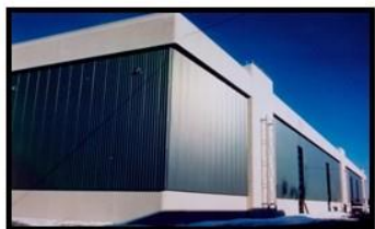
Solar Vent Air Preheat
