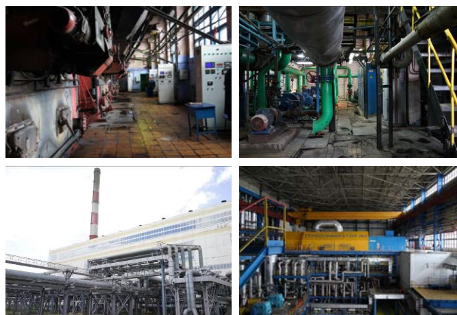
Fig 2.3.2 Boiler House(Top) and CHP facility(Bottom)
